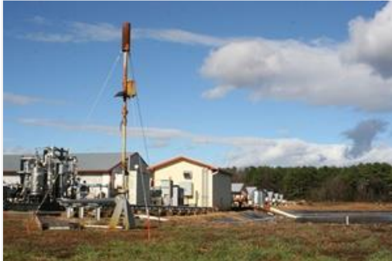
A flare burns leftover biogas to minimize methane
